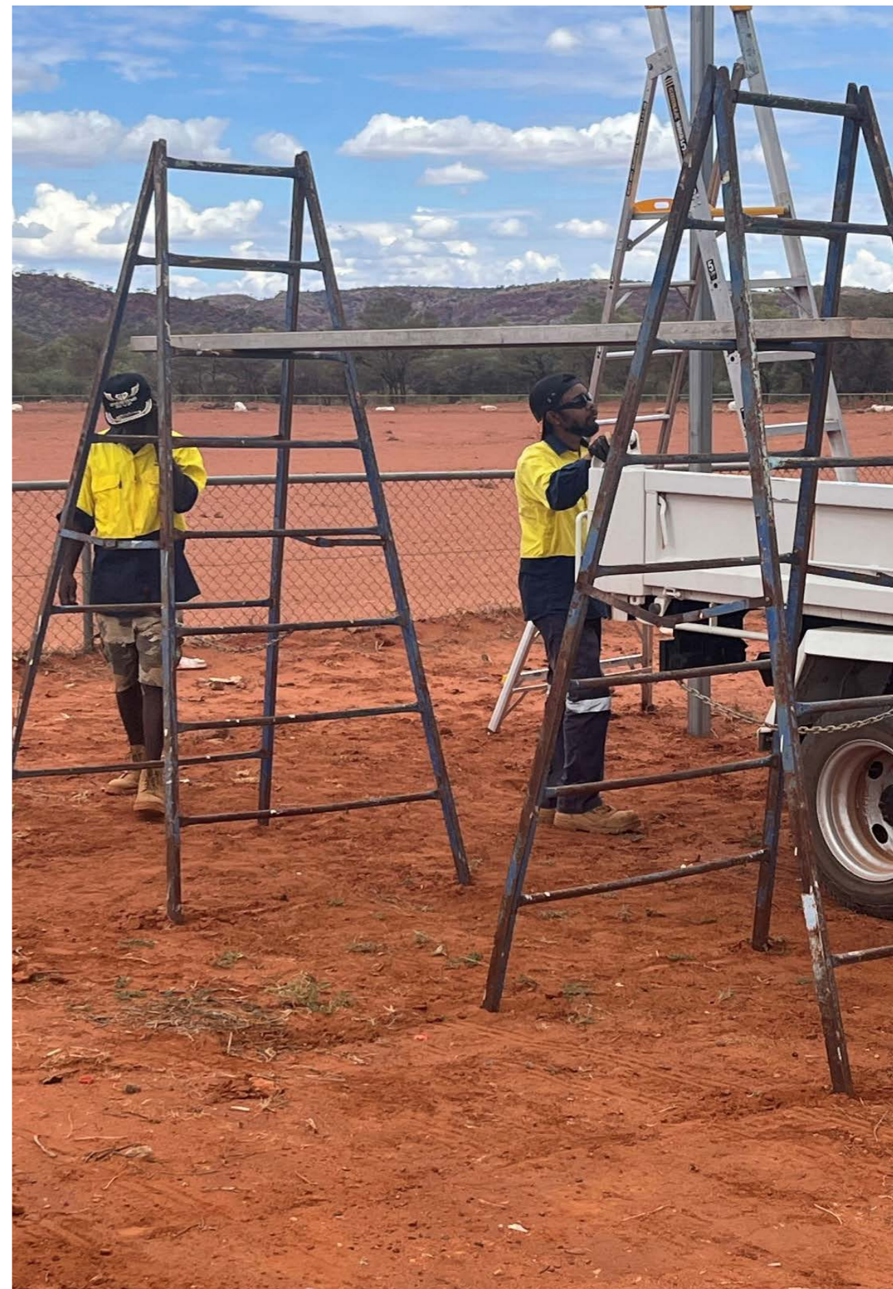
The Areyonga Civil Works Crew start work on erection of a shade shelter at the oval. The works were completed in 23-24
