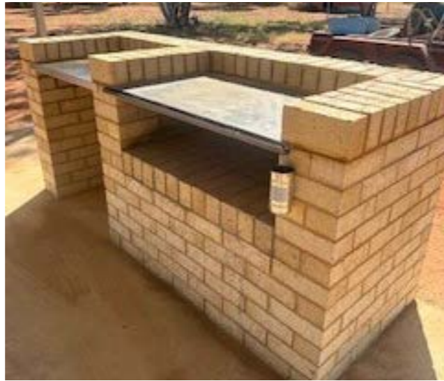
Warren Creek - Supply and installation of structures, lighting and wood fire barbecue
