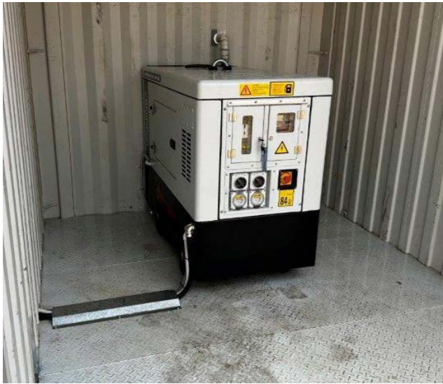
Green Valley - Supply and installation of generator
