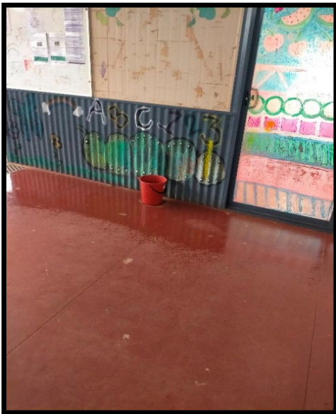
Some flooding in the childcare
