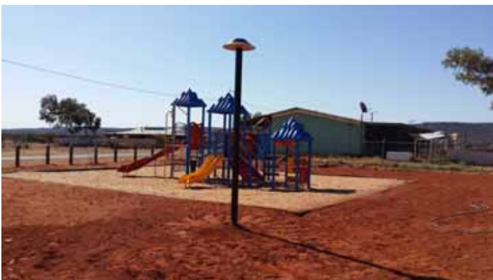
Solar bollard light installed Imanpa park
